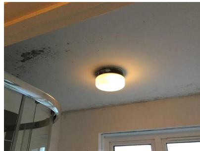
Bathroom ceiling showing mould no extractor fan installation of extractor fan would help
