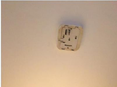
Hall smoke detector missing
