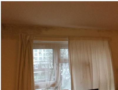
Mould appearing on bedroom three wall above window course needs investigating
