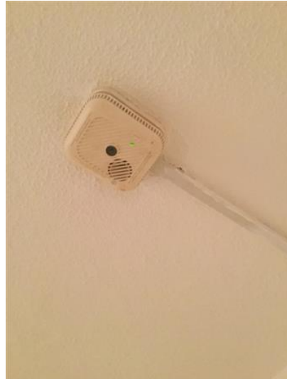
Landing smoke detector tested and working
