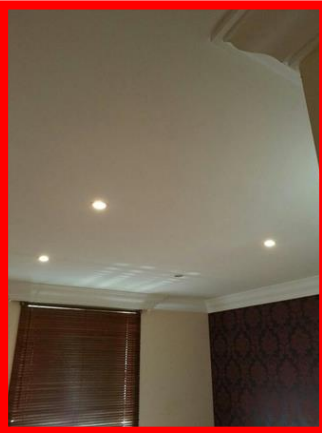
Four halogen spot lights. One not working.
