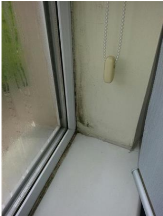
Some minor mould around window frame inside.
