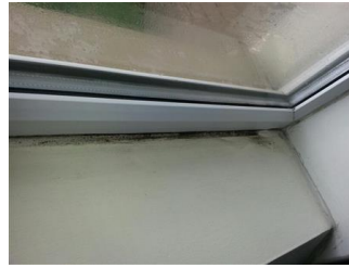
Some minor mould around window frames inside.
