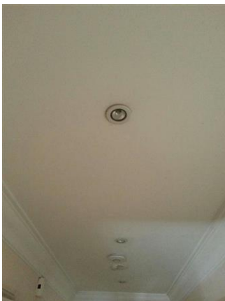
Three spot lights. Halogen. Two not working.
