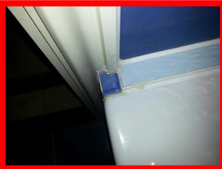
Loose tile to corner of bath.
